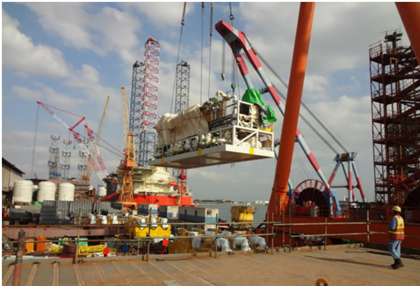
Photo bottom Cuttings reinjection unit (pump segment) being lifted onboard West Linus jack-up drilling rig.
