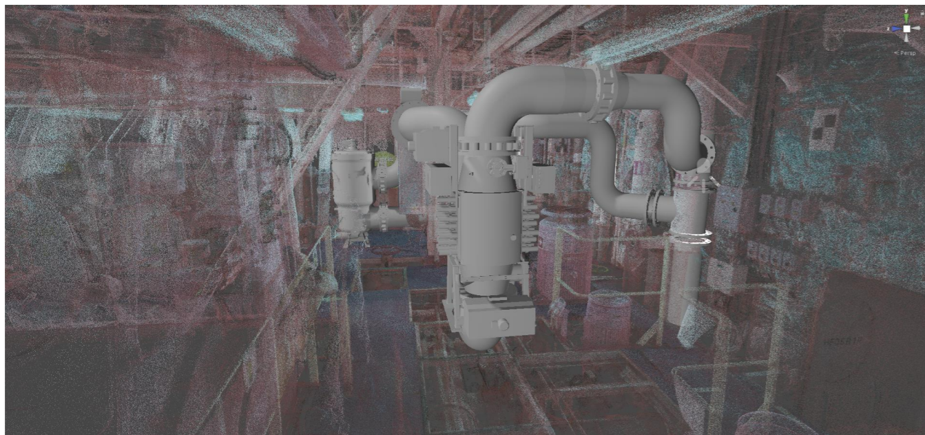
Photo below Point cloud scan data merged with 3D model of developed BWTS package installed within an engine room.
